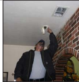
Technician checks the smoke detector at senior's home.
