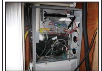
Central Heat Unit inspected and cleaned
